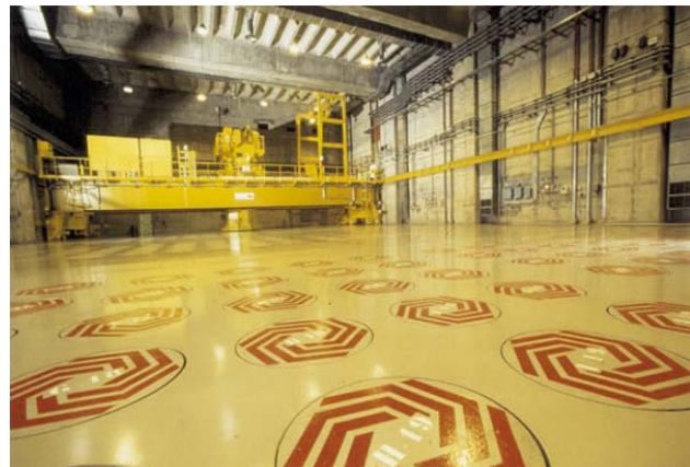
The France HLW storage facility
