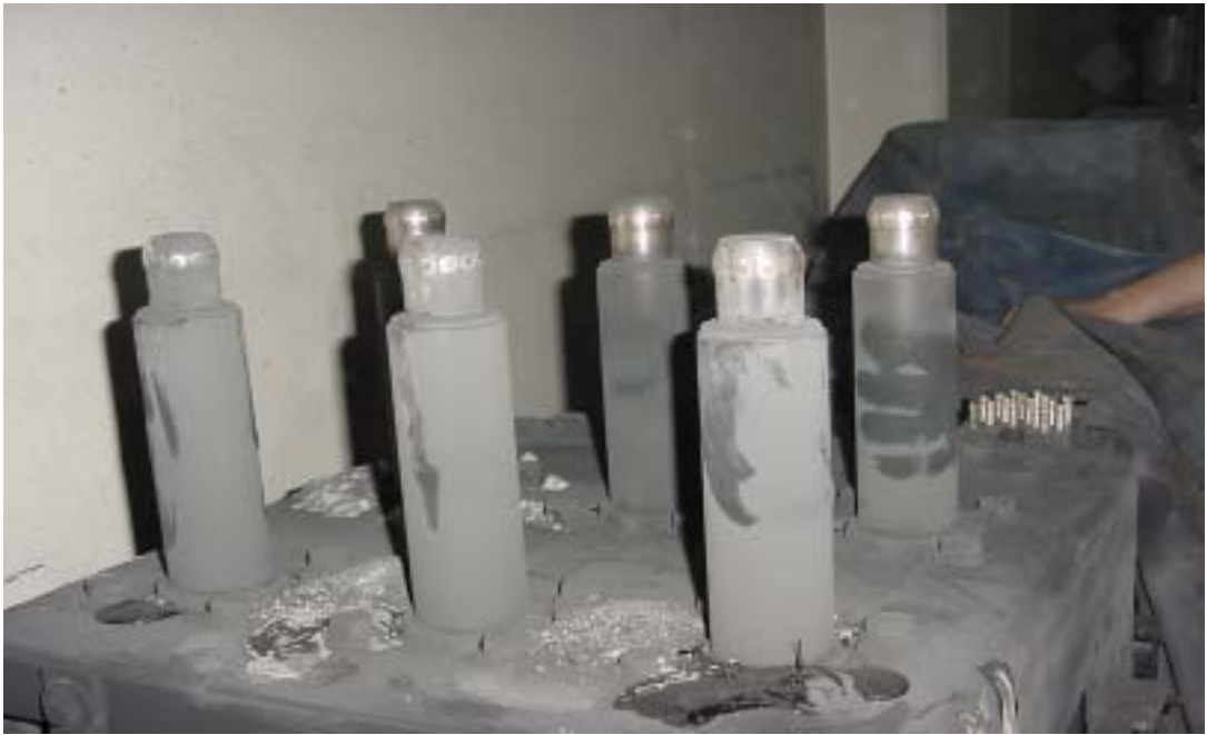
Connector damages of breaker #15
