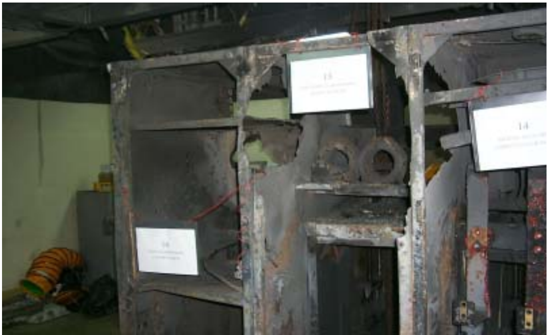
Damaged essential 4.16KV bus switchgear
