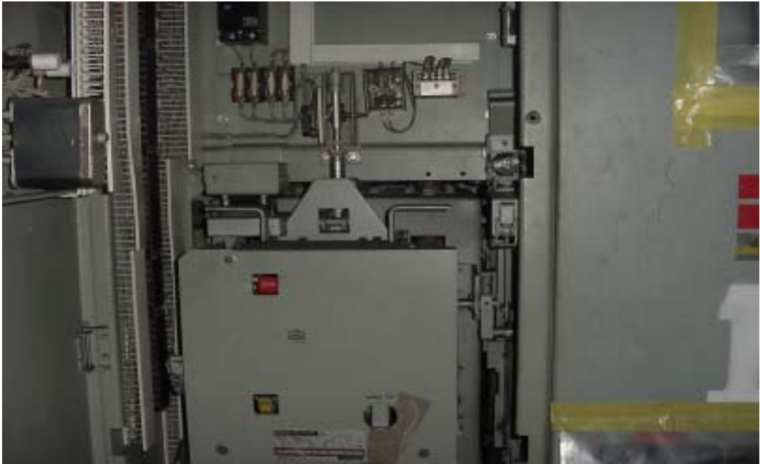
Appearance of a normal breaker arrangement at a switchgear
