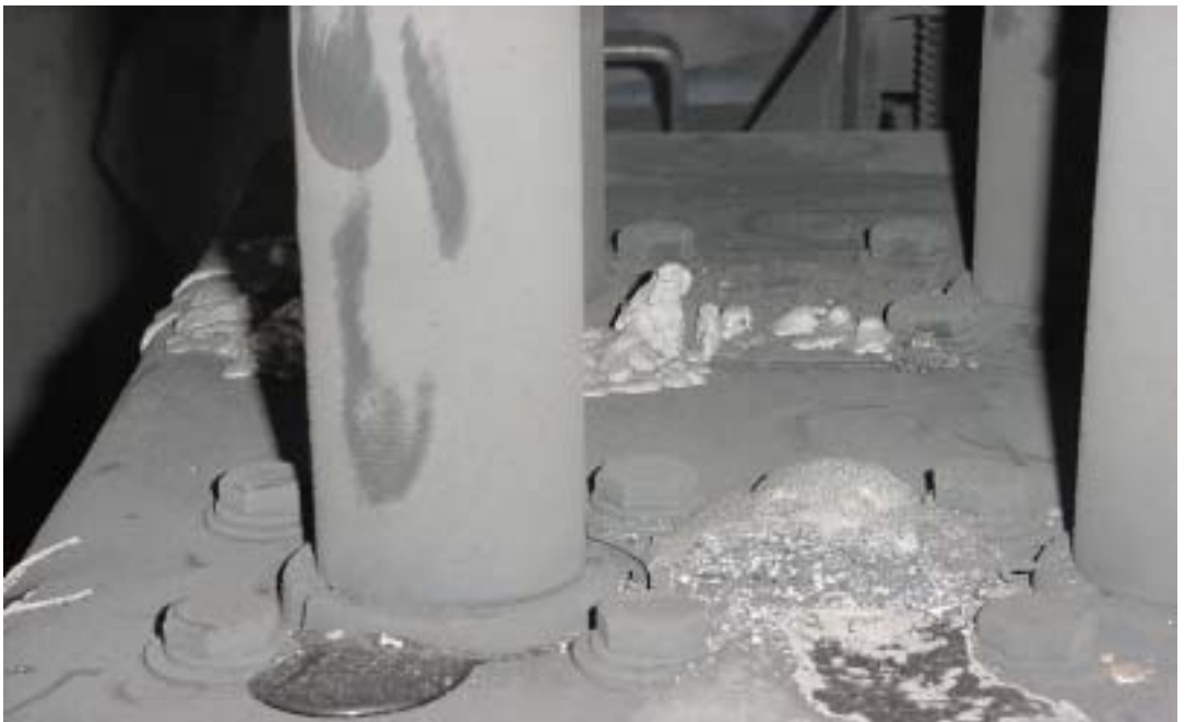
Frame damages of breaker #15
